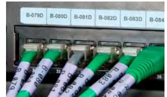
Patch Panel Labels
